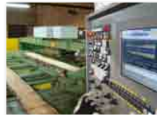
Operator control panel
